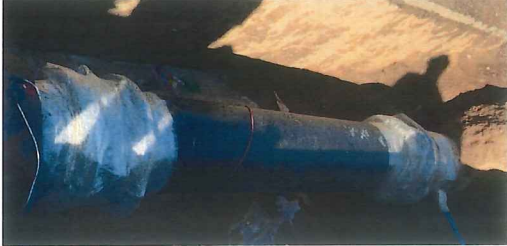
Poly wrapped pipe in D Street Bridge
